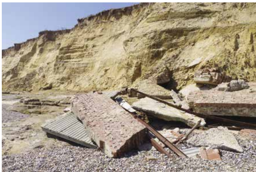
Collapsed buildings and exposed beach platform: Covehithe 7 weeks after the 'The Mini-Beast' (photo: S Brooks, 7.5.2018)
